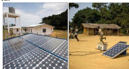
Figure 5. Solar Panels Generate Electricity in Liberia
